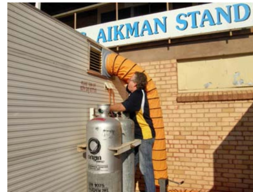
Phillip connecting the extractor for the Chip Van at the Grand Final
